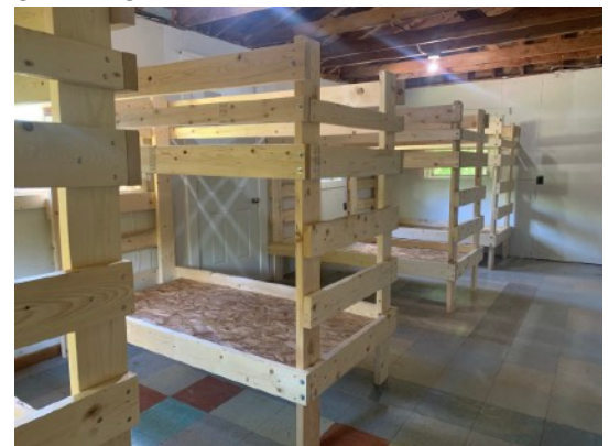
Our old director's cabin has been renovated into a new camper cabin! Thanks to Falmouth Baptist and Christ Community Church for sponsoring this project
